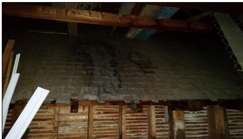
Part of the 1848 roof can be seen in the attic space of the 1895 addition.
